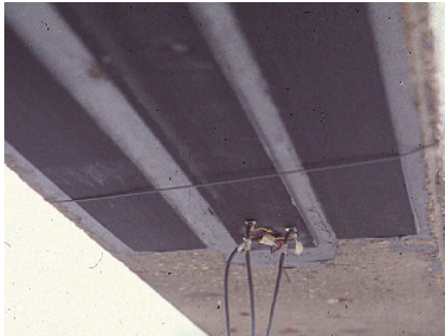
Figure 10 CFRP Plates bonded with epoxy to a concrete beam Image from http://www-civ.eng.cam.ac.uk/cjb/cjbresearch1.html
