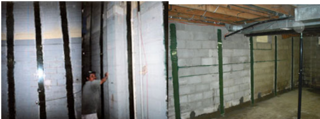
Images of carbon FRP plate (left) and carbon FRP grid (right) adhered to masonry walls for strength increase to resist bending loads
