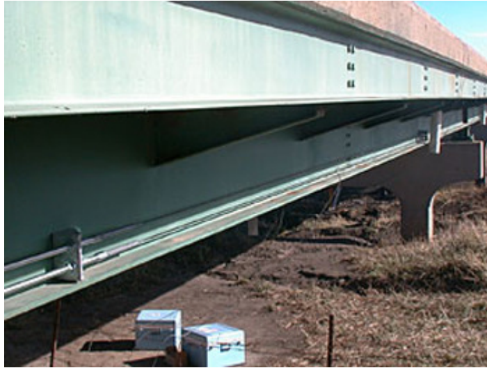
Photo of the Strengthening of Steel Girder Bridge Using Post-tensioned FRP Rods/Strands
