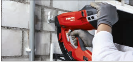
Conduits and light-duty pipes
